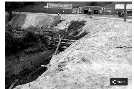
Circa 1936: Efforts to stabilize and widen Riverside Avenue in Burlington included a wooden grid structure and a great deal of sand and gravel fill, as seen in this photograph by L.L. McAllister. The Fairview Garage and gas station can be seen in the road's deep curve. SPECIAL COLLECTIONS, BAILEY/HOWE LIBRARY, UNIVERSITY OF VERMONT
