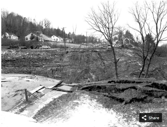
A massive 1955 collapse of the hillside beneath Riverside Avenue in Burlington closed the road and literally undermined decades of work to stabilize the slope. This photograph was taken Dec. 8, 1955 by James Detore to document damage for the American Fidelity insurance company.
