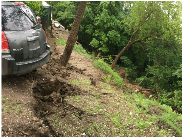
Figure 9: Soil cracks and slumping visible on the slope at the site of the 2019 landslide months prior to failure
