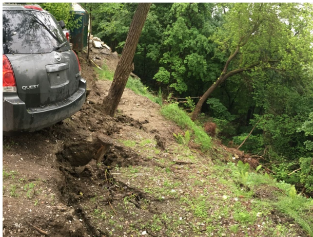
Figure 9: Soil cracks and slumping visible on the slope at the site of the 2019 landslide months prior to failure
