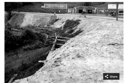
Circa 1935: Efforts to stabilize and widen Riverside Avenue in Burlington included a wooden grid structure and a great deal of sand and gravel fill, as seen in this photograph by L.L. McAllister. The Fairview Garage and gas station can be seen in the road's deep curve. SPECIAL COLLECTIONS, BAILEY/HOWE LIBRARY, UNIVERSITY OF VERMONT
