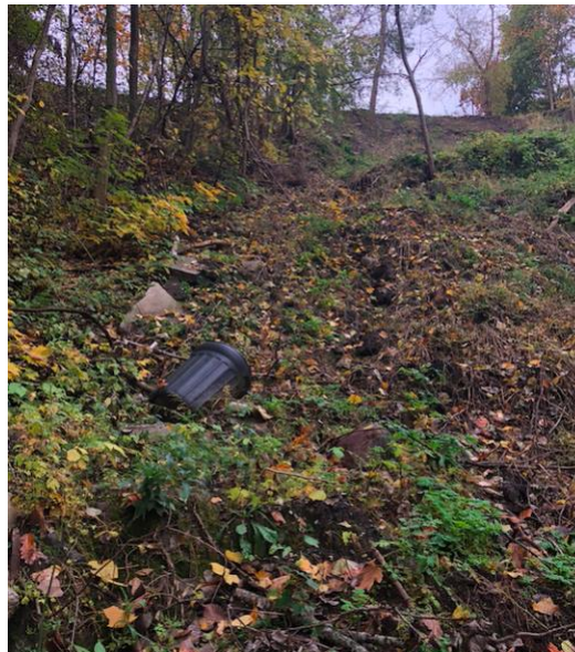
Figure 2: Image of the steep slope where the 2019 landslide occurred. Various debris including trash and concrete are visible.
