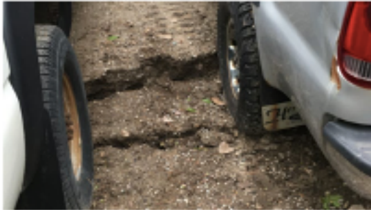
Figure 5: A 6-inch gap begins to form, cracking shortly before the 2019 landslide occurred (Paul Bierman 2019).
