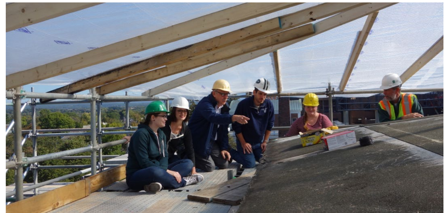
(Below) Professor Thomas Visser points out historic roofing features on Torrey Hall to UVM historic preservation graduate students with Scott O’Brien (right) of UVM Physical Plant, who discussed various technical challenges.
