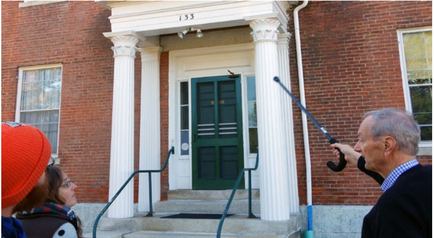
Henri de Marne points out moisture issues visible on the side entrance to Wheeler House, the UVM Historic Preservation Program's headquarters, built in 1842.
