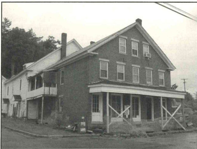
Rehabilitation of the Harrisville General Store in progress; Harrisville, NH. (Erin Hammerstedt)
