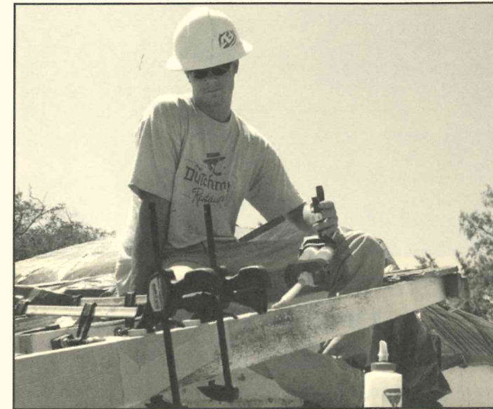
Joe Haun conducts an epoxy pour on a rafter in situ at the Las Flores Adobe Ranch House.
