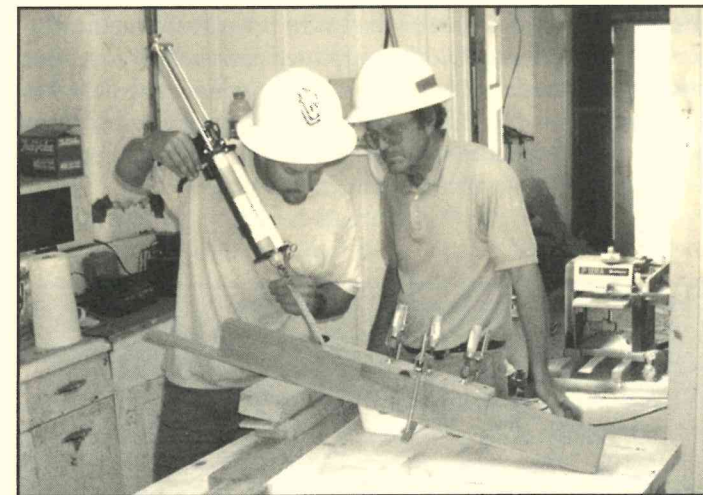
Eliot Lothrop and Jake Barrow, NPS senior exhibit specialist, conduct an epoxy strength test at the Las Flores Adobe Ranch House.
