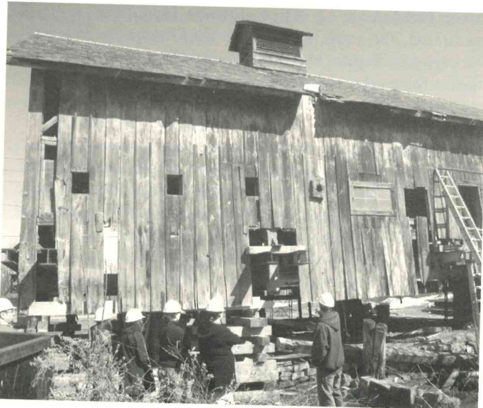
Eliot Lothrop, '03, shows Historic Preservation students his recent project rehabilitating a barn in the Intervale, Burlington, Vermont. This rehabilitation was part of a larger project to move the barn across the road for adaptive reuse by the Intervale Foundation.
