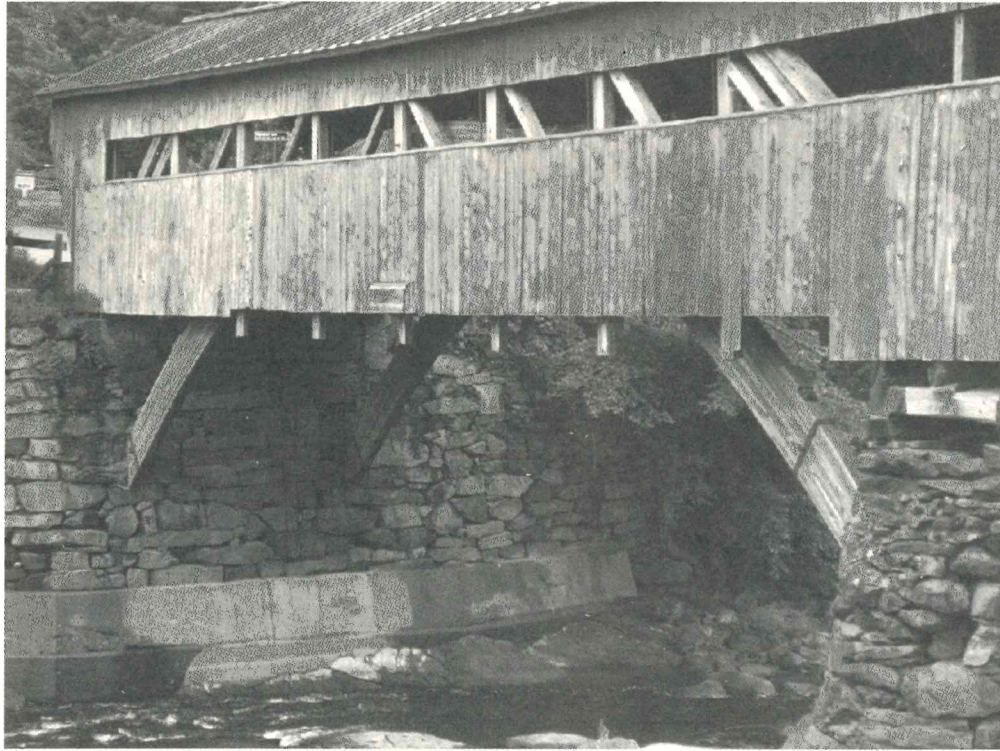
Covered bridge built in Taftsville, Vermont, 1836: Truss system comprised of King Post, Queen Post and arches with iron rods (photograph by Roger Ciuffo for Covered Bridge Project 2004: see article on page 6)
