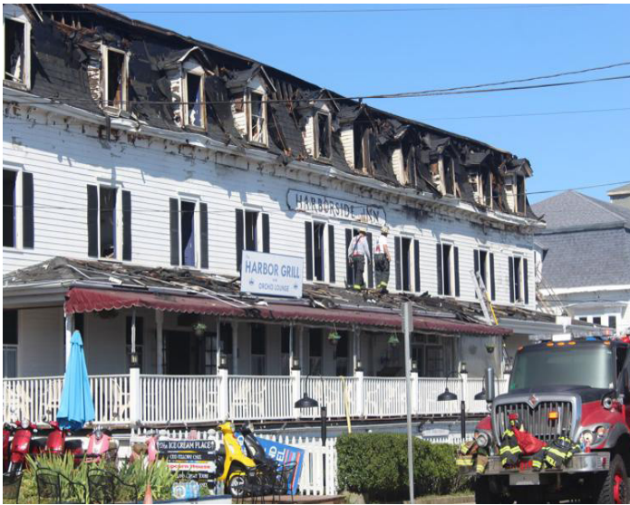
The Harborside Inn on Block Island, RI, following a fire on August 18, 2023. Photo courtesy of The Block Island Times.
