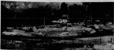
EMERGENCY ROAD BYPASSES RIVERSIDE AVENUE WASHOUT—Sunday traffic was new asphalt. New pavement was built in a loop through the city ball-dump property and enables normal flow of traffic along Riverside avenue. Reconstruction of the main road is expected to cost about $35,000 with the state footing 70-80 per cent of the bill, according to Mayor J. Edward Moran.
