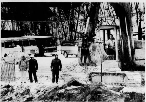
Alan Pidgeon, Mike Colby and Roger Atkins, left to right, watch as backhoe operator Bob Grant begins to build a work road to be used during construction to correct an
